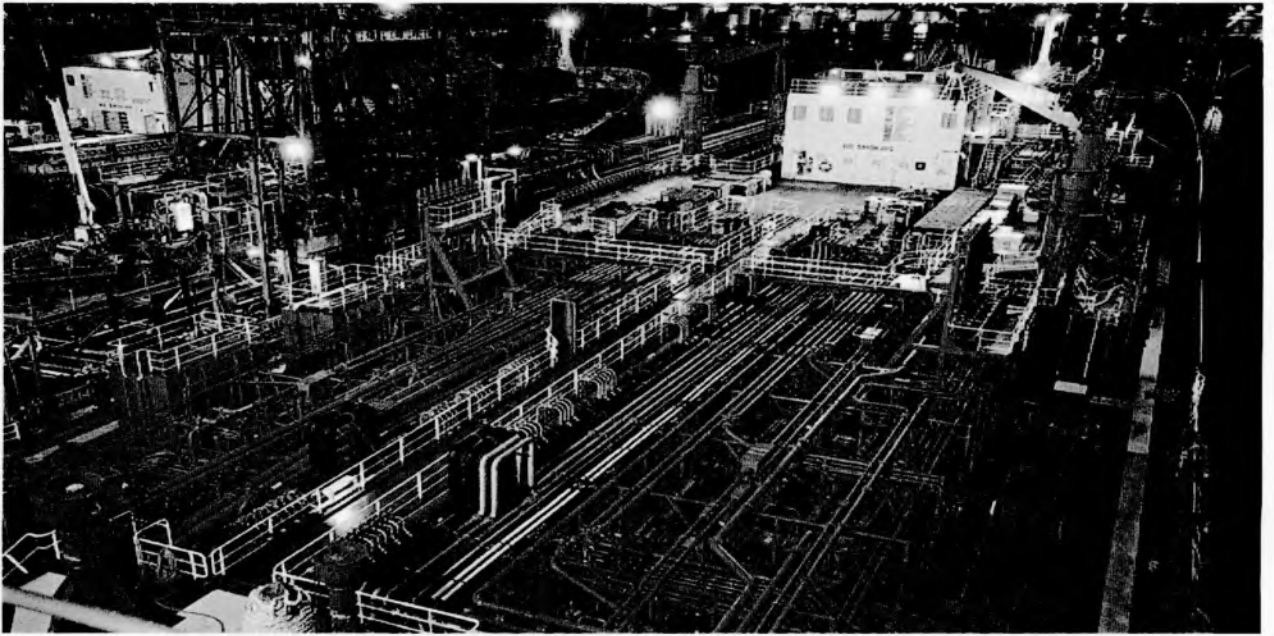
Figure 1.3.2 C – Chemical tanker deck pipeline arrangements
